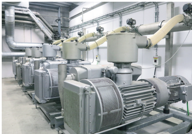
The pump room showing installed R 5 rotary vane vacuum pumps.
